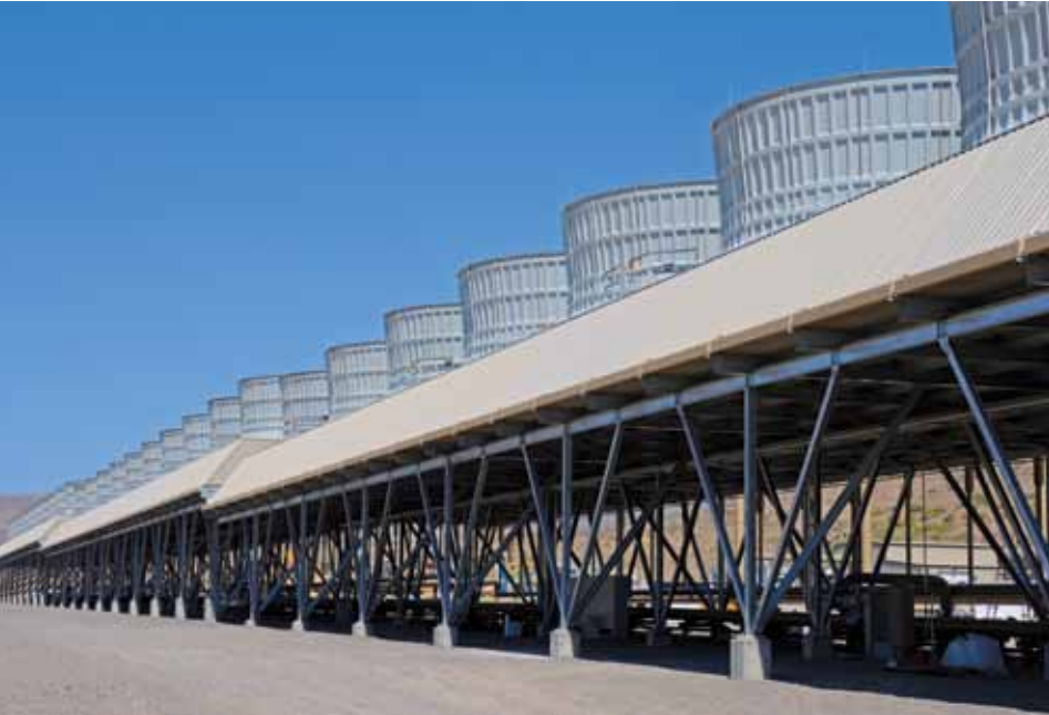
U.S. Geothermal began commercial operation of the Neal Hot Springs 22 MW facility in November 2012. With 30, 100 HP condenser fans, this is the company's newest and largest plant.
