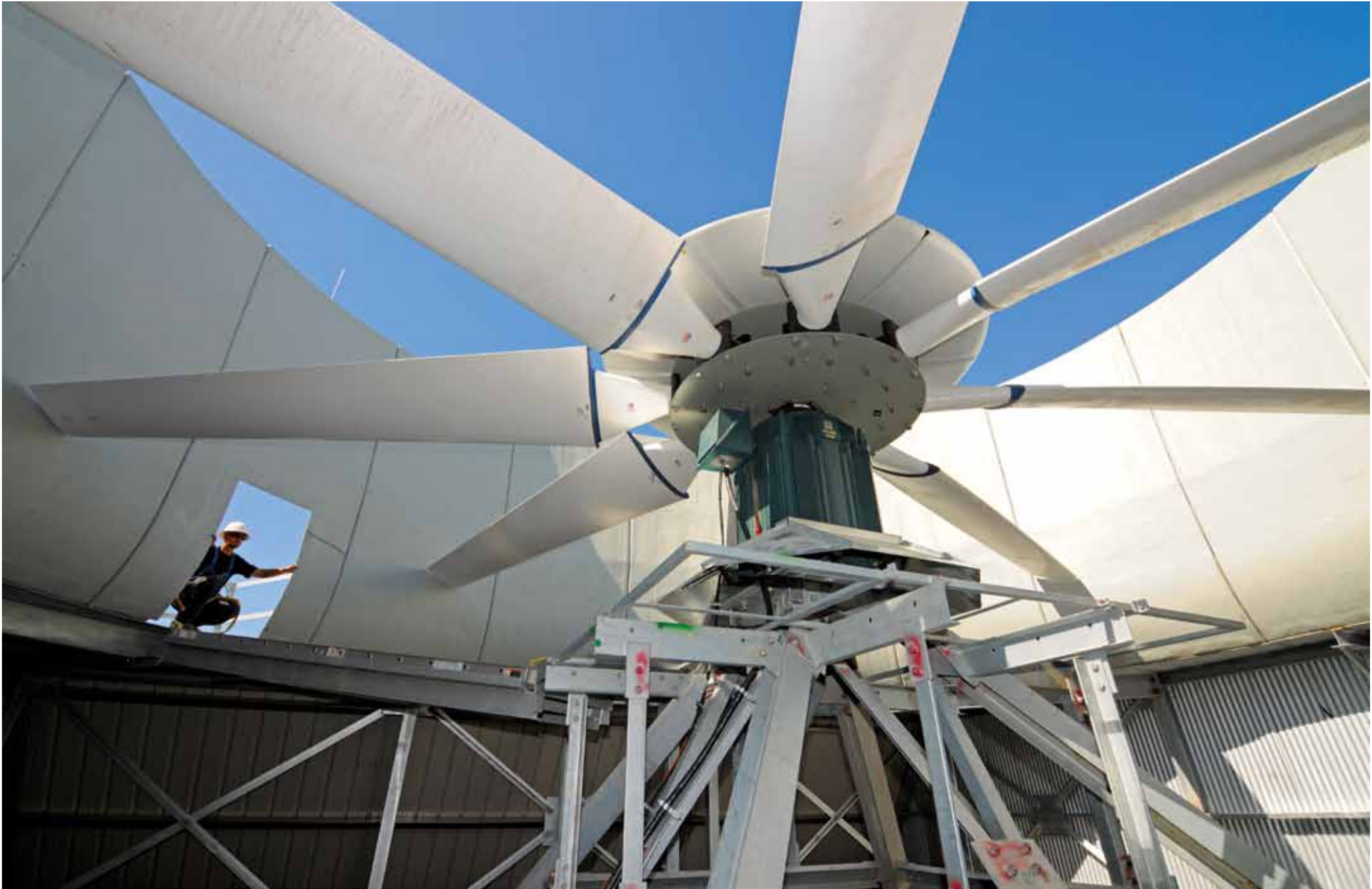
U.S. Geothermal was the first company in the geothermal industry to adopt Baldor’s cooling tower motor solution for air-cooled condensers. Kevin Kitz, the company’s VP of project development, says the advantages of using the Baldor solution are crystal clear, calling it a very efficient motor with very low maintenance costs.
